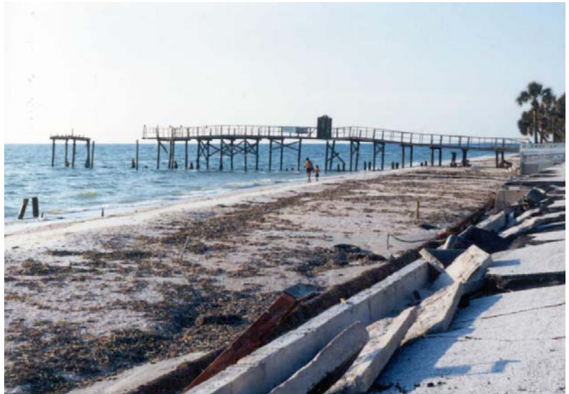
Storm damage during the 1980's. The big pier was condemned. The storm exposed and broke-up the original roadbed on the beach.
